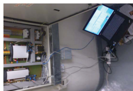
Fig. 17. Wireless deployment (picture left rotated)
